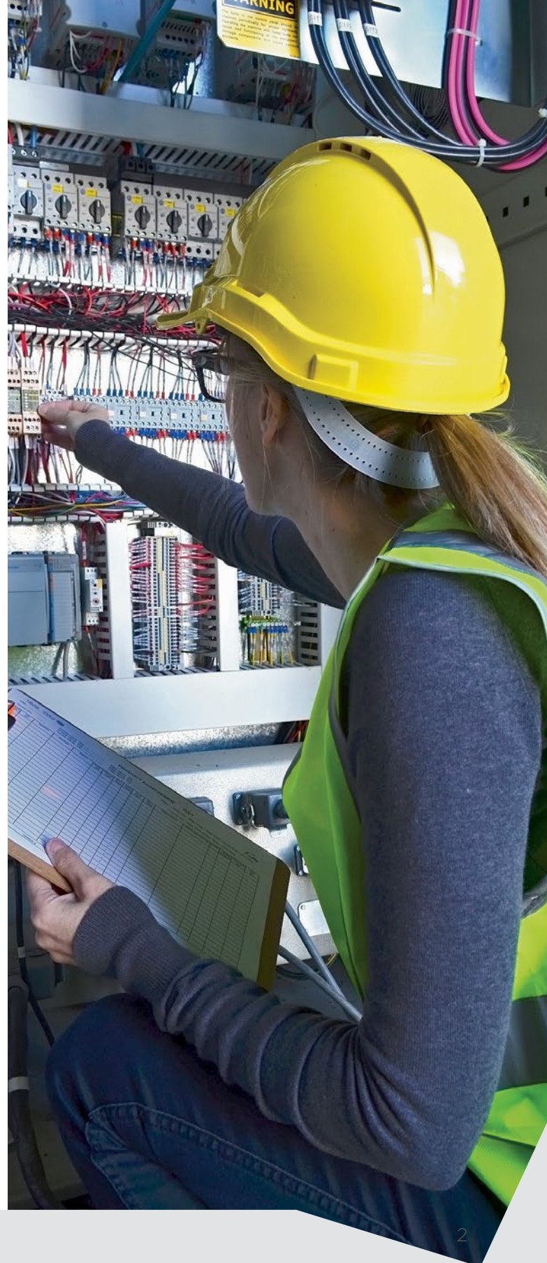
Voltage optimisation (credit: iStock)
